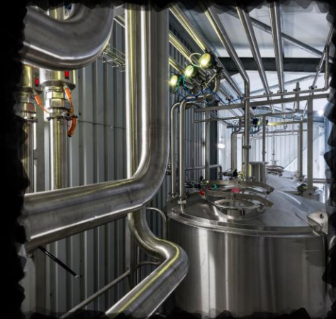
✓ CIP (Clean in Place)
