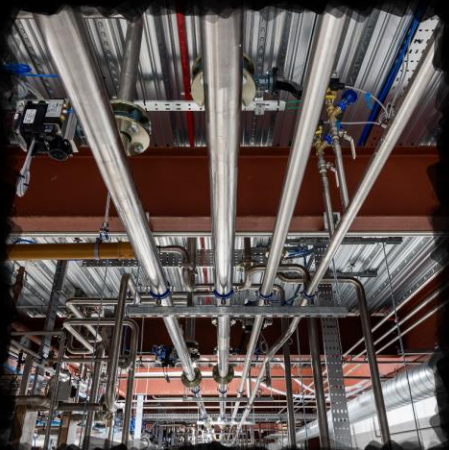
✓ Hygienic/ Service Pipework
