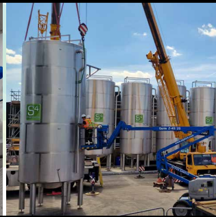
Storage, Holding, & Transfer
